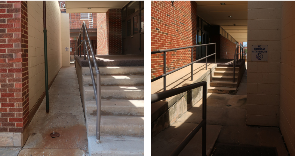
ACCESSIBILITY ISSUES AT ENTRANCES
