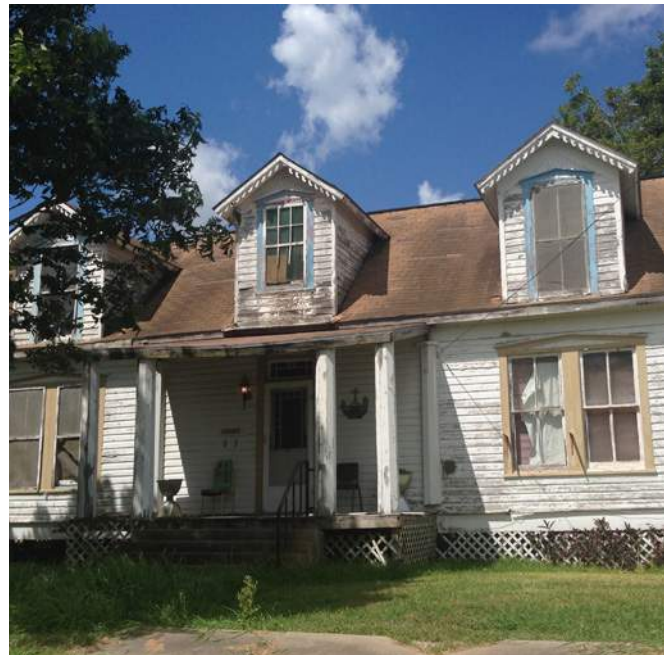
Planning for incremental redevelopment can help ensure that as properties age and deteriorate like this, regulations make it easy to replace them with modern, high quality housing stock.
